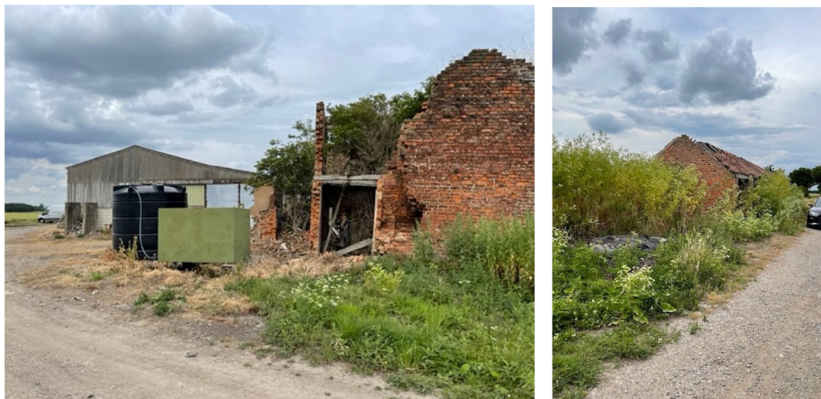
Figure 3-6. Dilapidated dwelling and modern barn at Johnson's Farm
